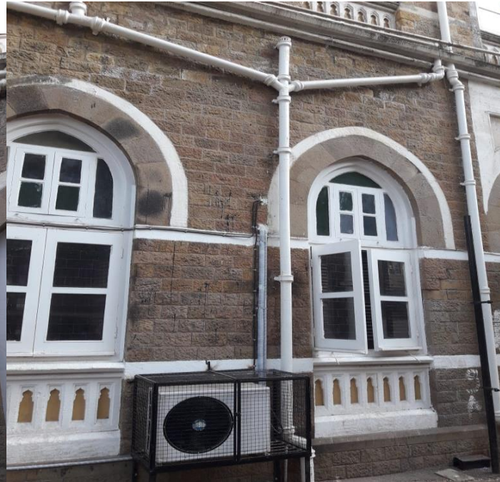
Network of pipes
